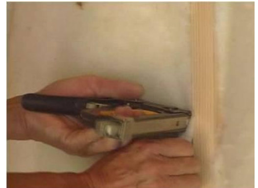
When stapling the insulation into the stud wall, it is important to allow clearance for the plaster board
